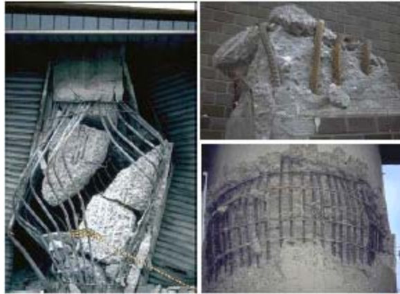
Figure 7-3: Column failures in Kobe 1995 earthquake (EQE 1995).
