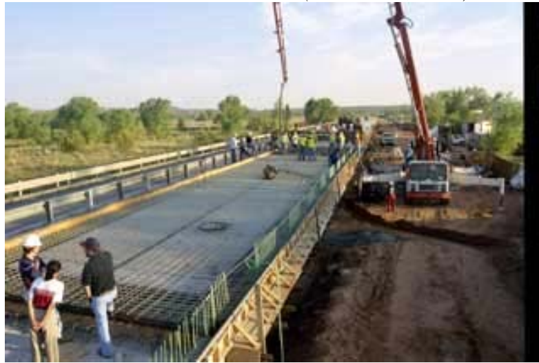
Figure 8-1: Use of GFRP rebars in construction of Sierrita de la Cruz Creek Bridge, RM1061 Amarillo Texas (Aslan FRP, 2004)
